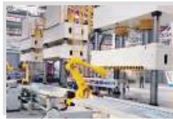
冲压上下料 Stamping loading and unloading
